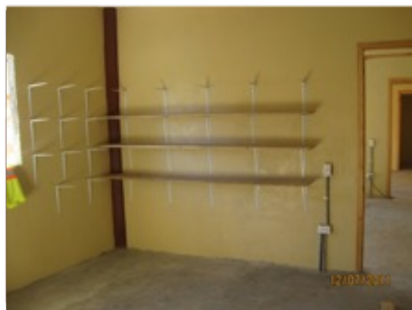
Every consultation room has a sink and cabinet. The pharmacy room has shelving around the whole perimeter with a desk in front of the window to serve patients.
