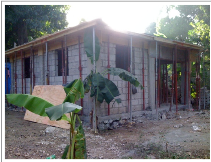
↑ The houses are formed with lumber and shores for the concrete roof.
